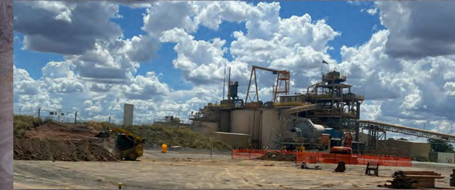
MACA Interquip awarded refractory upgrade design, engineering and construction contract at Tomingley Gold Operations, New South Wales, Australia
